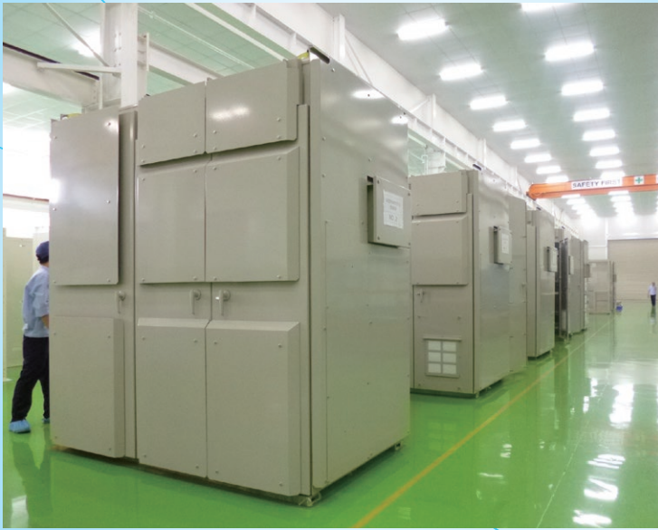
Power conditioner enclosure
