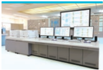
Supervisory Control System for Waterworks
