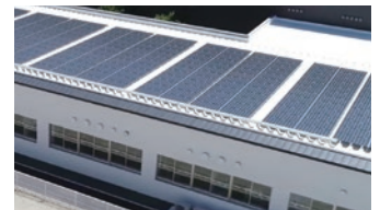
Photovoltaic system installed at the Nissin Academy Training Center
