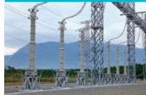
550kV Capacitor Voltage Transformer
