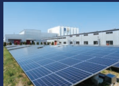
Captive Consumption Photovoltaic System
