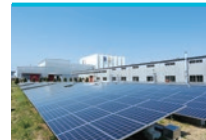
Captive Consumption Photovoltaic System
