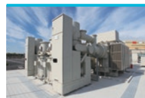
77kV Extra-high Voltage Substation Equipment
