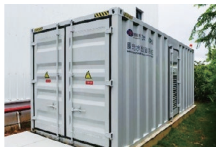
Membrane water treatment equipment
