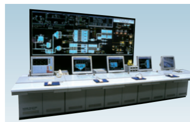
Supervisory Control System for Waterworks
