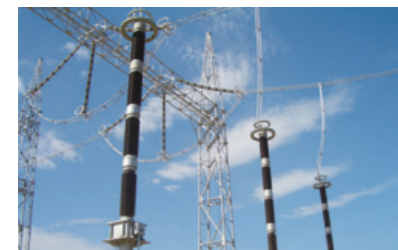
Capacitor Voltage Transformer (CVT)
