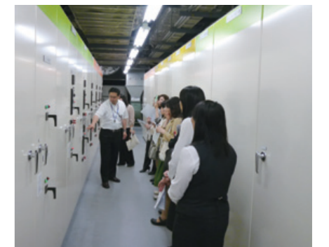
Visit to sites installed with Nissin Electric products
