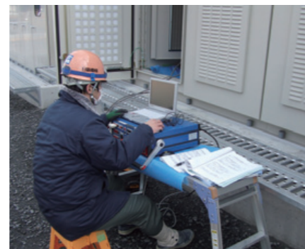
Site test being made on a power conditioner
